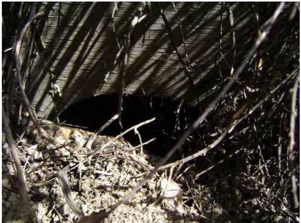
Photo 10. Drainage 3 also flows west to east down towards the I-15 corridor and is generally 2 foot wide. This partially blocked 48-inch culvert is located at the downstream end of the channel near the shoulder of I-15.
