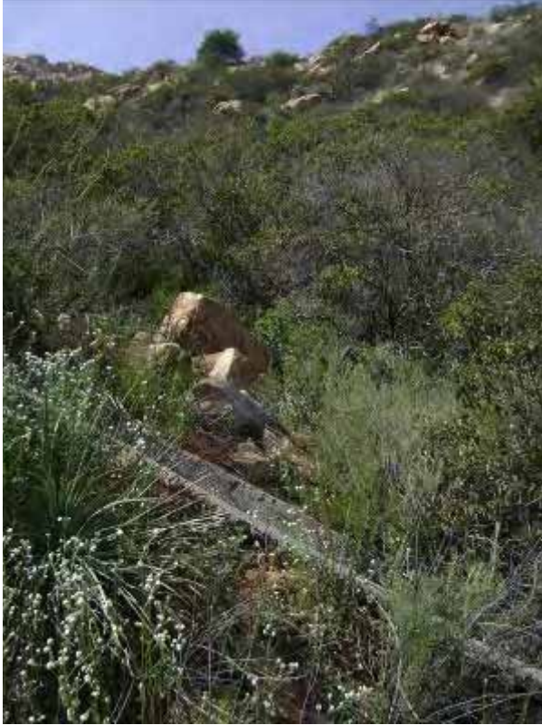
Photo 13. A concrete brow ditch that diverts sheet flows on this slope into Drainage 5. The channel is generally 1 foot wide and relatively short, and occurs under dense chaparral.
