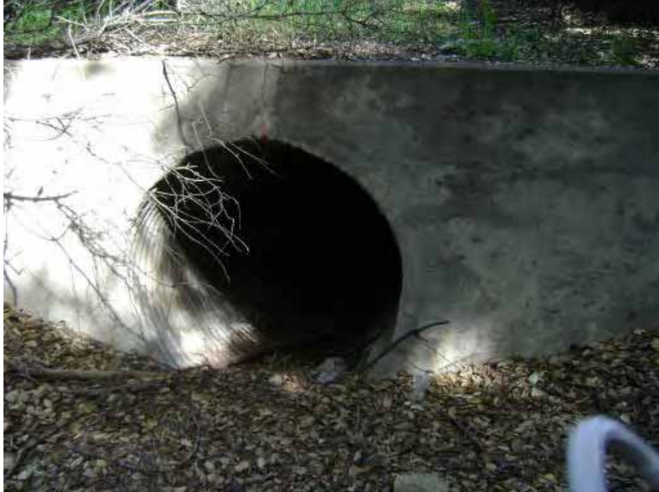
Photo 6. Drainage 1 flows west to east down towards the I-15 corridor and is generally 1 foot wide. This 36-inch culvert is located at the downstream end of the channel near the shoulder of I-15.
