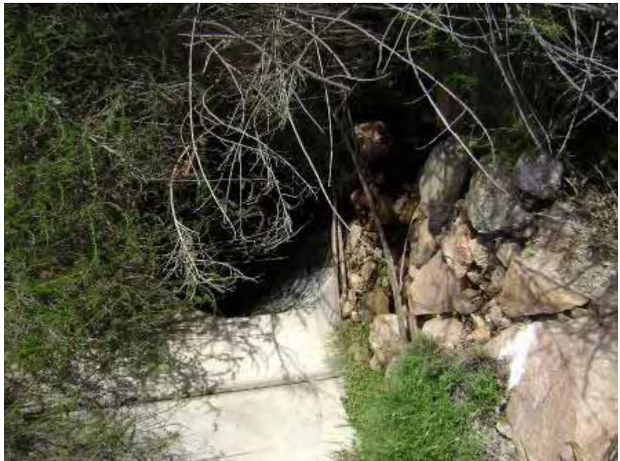
Photo 14. A 12-inch storm water inlet located at the downstream end of Drainage 5.
